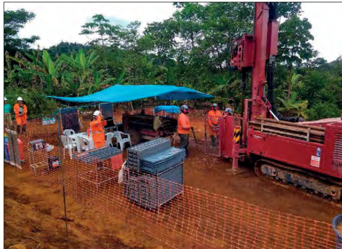
Figure 4. Sonic rig set up and safe drill site display. Gravel chips placed around rig working site prevent slippage.
