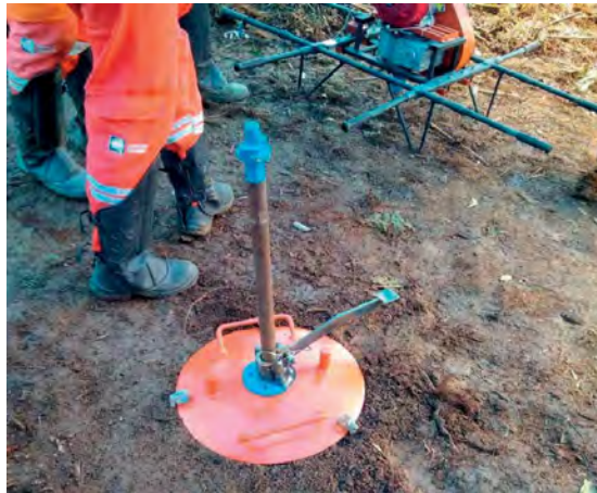
Figure 2. Auger site set up with bubble levelled metal collar protector in place. This is positioned after first meter completed (A horizon/organic material). Foot hold allows drilling down to 30 m.
